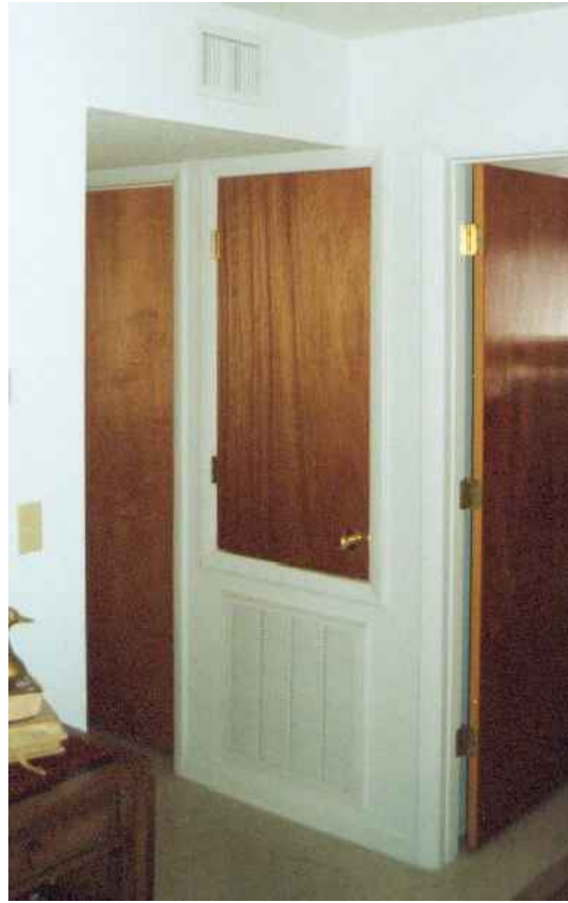
SHORT DOOR AT HALL CLOSET (DONT PAY ATTENTION TO THE WOOD DOORS & VENT!)
